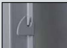
Main door latch hooks welded to frame
